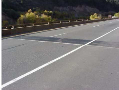
The bridge joints along I-70 in Glenwood Canyon are subject to high traffic loads and extreme temperature changes.
